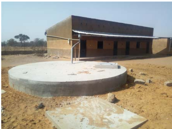
Figure 10.2 Rainwater harvesting system in Dekhaye School. (S.Sene, 2018).
