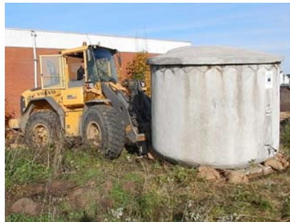
Figure 18.16 Town transport of a 6000 L Calabash Cistern. (Source: Author's own).
